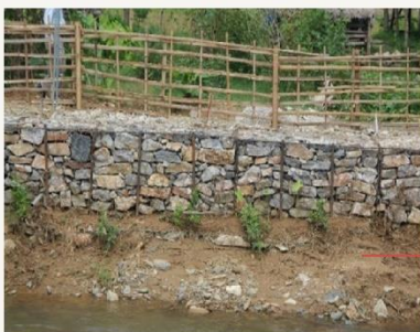
Vegetated Gabion Plants growing through layers of rock in vegetated gabion technique at riverbank embankment at SP32 in Son La Province, providing flexible binding to the structure once the wire has corroded - ICEM, 2017
