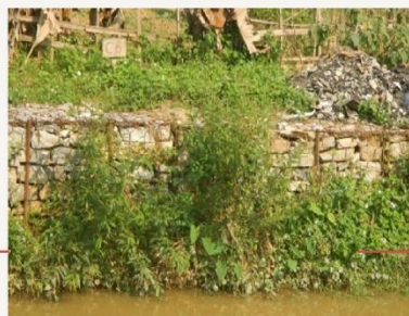
Vegetated Gabion Vegetated gabions in riverbank embankment at SP32 in Son La Province after one year and two flood seasons - ICEM, 2017
