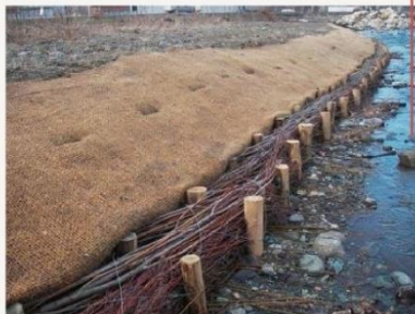
Vegetative geotextile including fascines and live stakes. Stenlund, et al. 2005. Minnesota Soil Bioengineering Handbook
