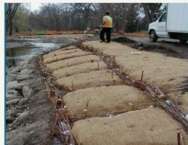
Vegetative geotextile including fascines and live stakes. Stenlund, et al. 2005. Minnesota Soil Bioengineering Handbook
